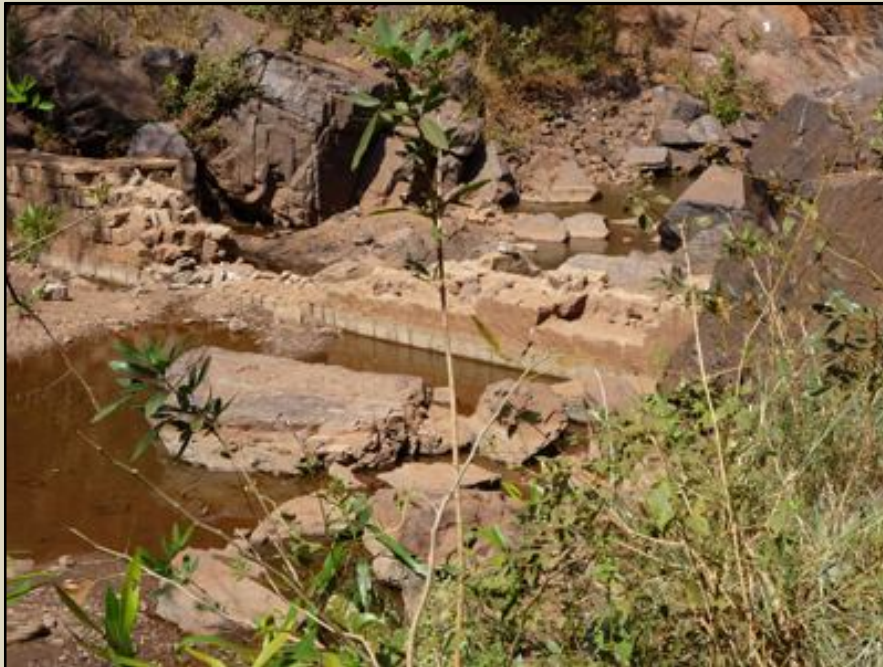
The check dam on the nulla within the MPCA is broken
